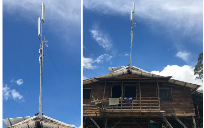
Figure 1: Tower installed on the local school’s roof, reusing existing infrastructure. This CoLTE site is able to cover the entire community from a single location.
