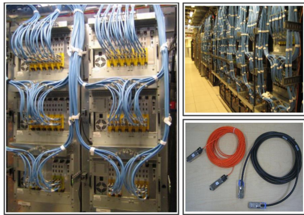
Figure 7: Two Firehose racks (left), each with 3 chassis with bulky CX4 cables from remote racks. The top right figure shows an aisle of cabled racks.
